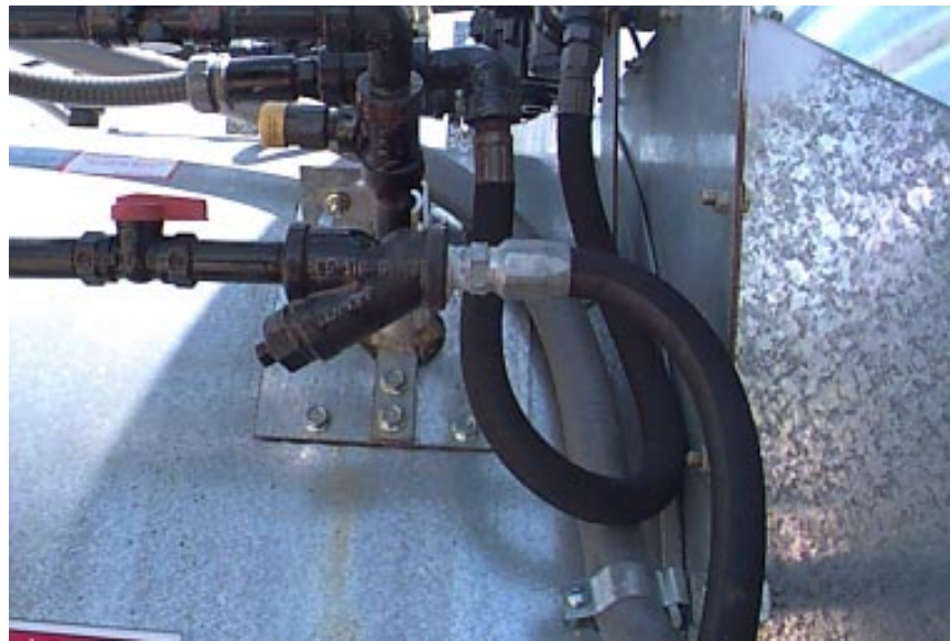
LP line field connection.
